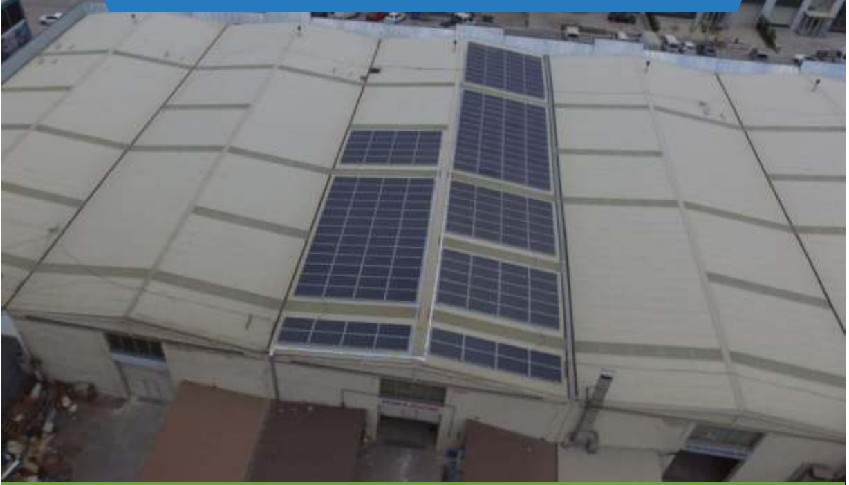
Dima Mermer | 87 kWp | KONYA - Karatay
