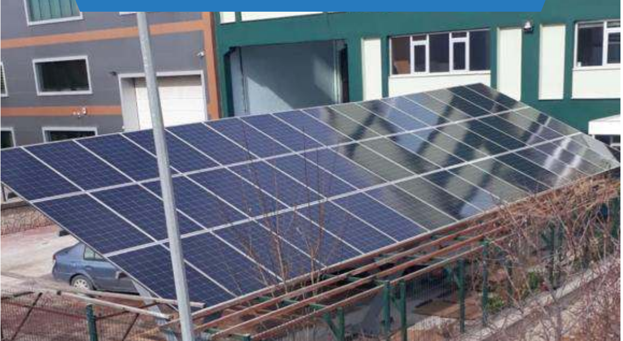
Apsan Otopark | 15 kWp | KONYA - Karatay
