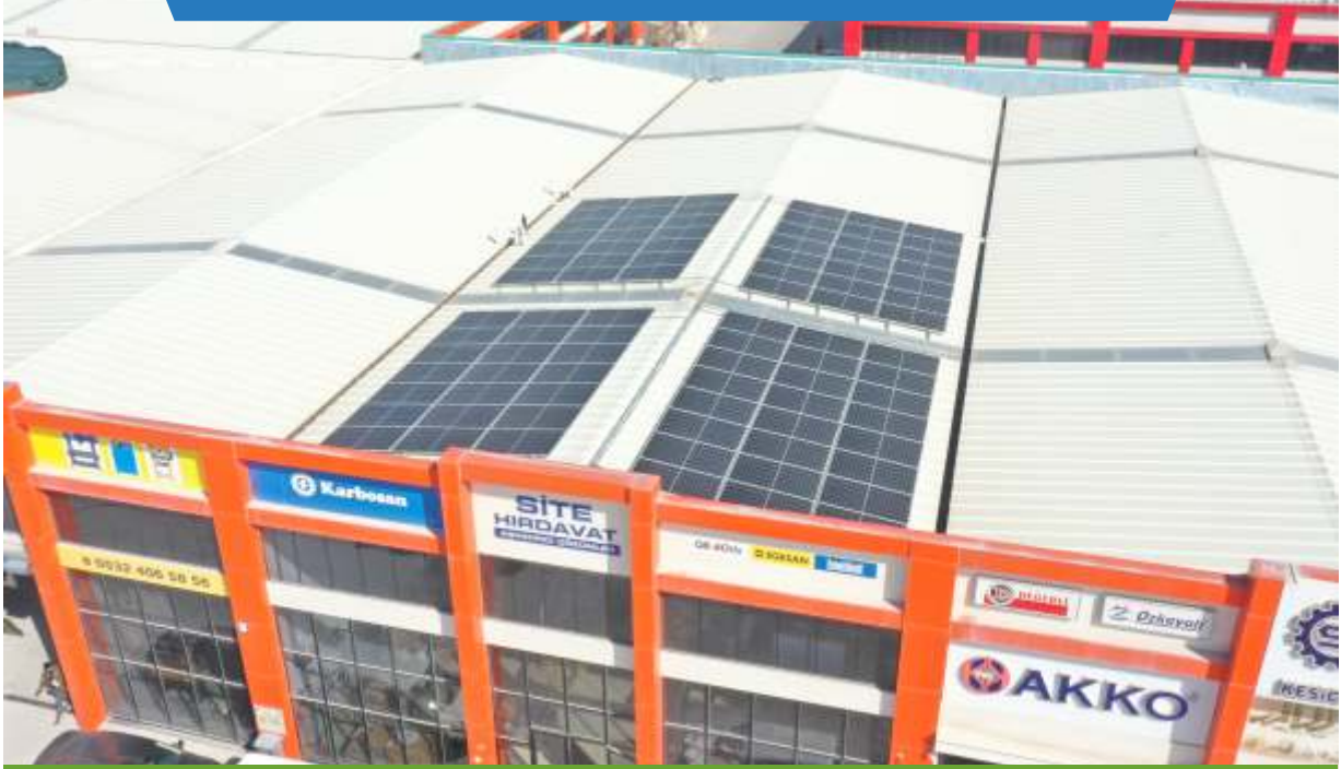
Site Hirdavat / 40 kWp / KONYA - Karatay
